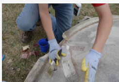
Figure 5. After cleaning and sanding the surface, cracks and the damaged edge of the dish were repaired using fiberglass cloth and automotive fiberglass resin. While at Bell Observatory, the steel support hardware was measured and inspected for bends and corrosion.
